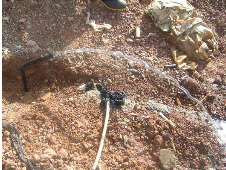
Plate 2: An illegal connection made onto the network
