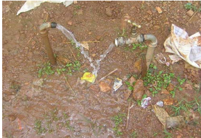
Plate 4: Typical example of a suspected illegal connection
